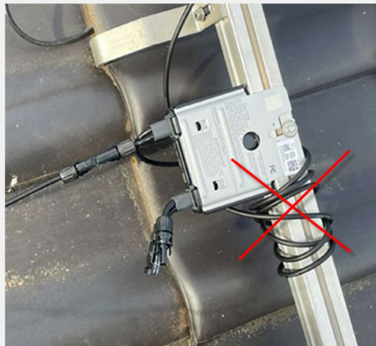
Figure 9: Example of an Incorrect Wire Loop
